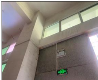
External photo(s) of the production unit(s) Exit sign and emergency light.JPG
