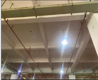
External photo(s) of the production unit(s) Sprinkle system.JPG
